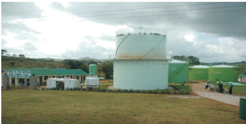
Katani's Bio-Gas plant at Hale
